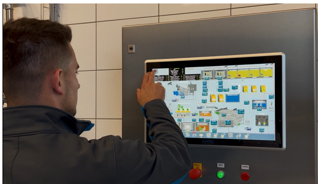
HMI panel in a wastewater treatment plant.
