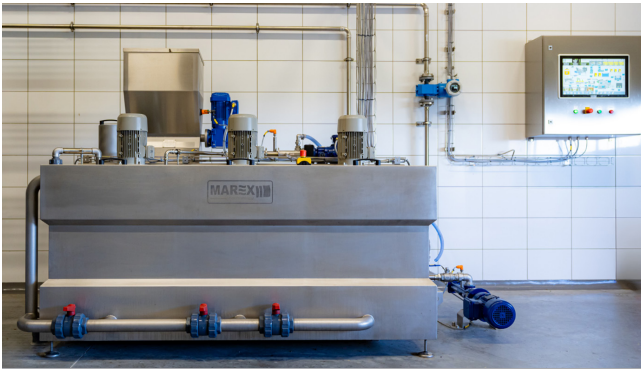
Polyelectrolyte station with control panel
